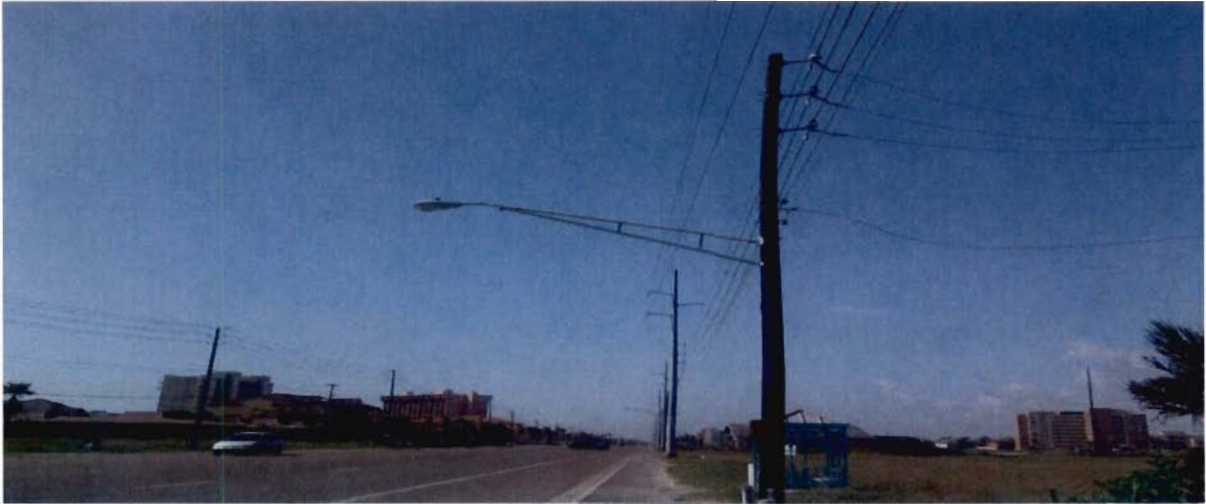
14' Arm with 250 HPS Lighting
