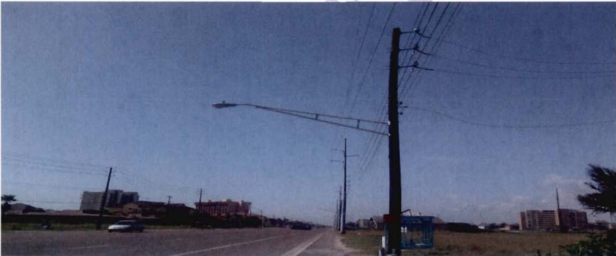
14' Arm with 250 HPS Lighting
