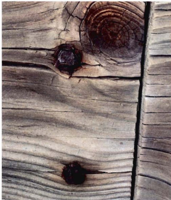
Photo #6 Advanced Nail Corrosion
