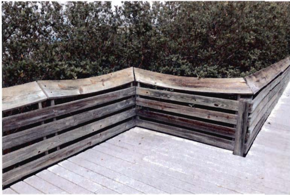
Photo #3 Warped Top Rail Member at Boardwalk Bend
