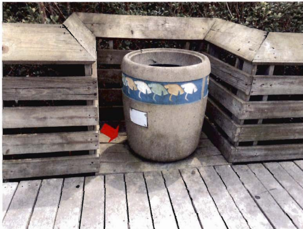
Photo #4 Walking Deck Surface Deflecting Under Trashcan
