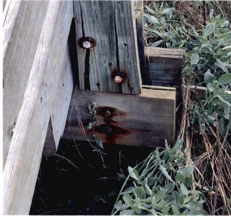
Photo #1 Advanced Splitting at Through-Bolt Connections. Replacement of Guardrail Post Member Shown.
