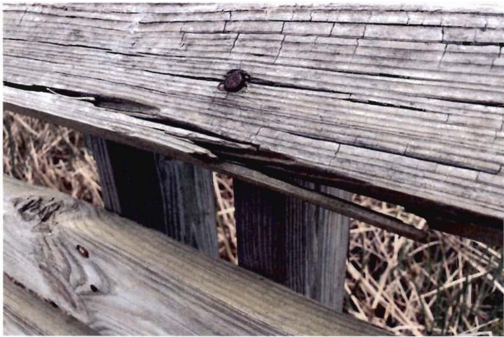
Photo #5 Top Rail Splintering & Advanced Nail Corrosion
