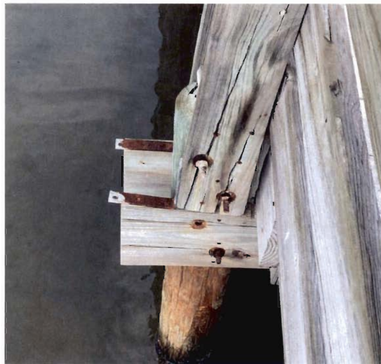
Photo #2 Advanced Splitting at Through-Bolt Connections. Replacement of Guardrail Post Member Shown.
