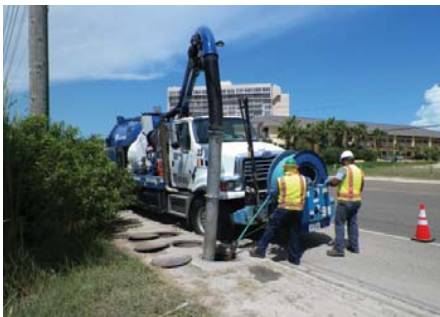
(Above) Storm Sewer Cleaning Laguna Madre Water District is contracted with the City to clean city storm drains: Completed 9/18/12
