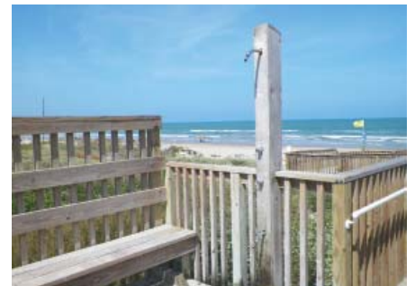
Vandal Proof Showerheads Installation of vandal proof showerheads at beach accesses: Completed 7/11/12
