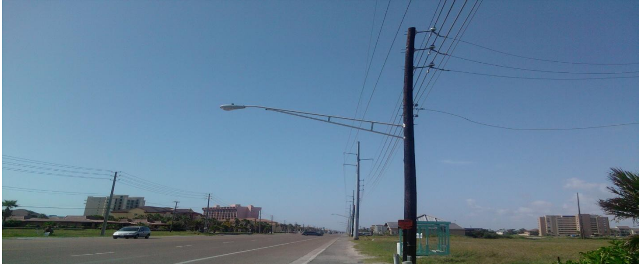
14' Arm with 250 HPS Lighting
