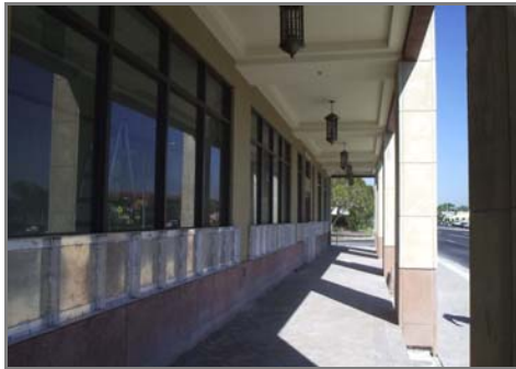
Example of Dry Flood Proofing removable panels utilized in a Bank Building in Naples Fl. – Appropriate in the Bayfront, Entertainment District Core, Neighborhood Crossing, and Town Center Crossing Zones
