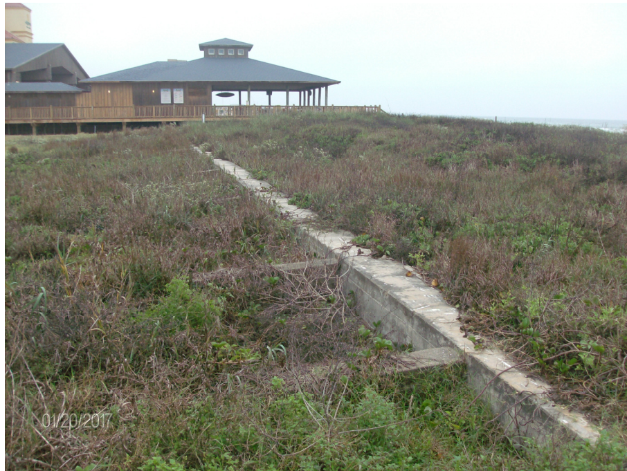
View of existing Bulkhead facing north (vegetation will be mitigated to the east of the proposed bulkhead)
